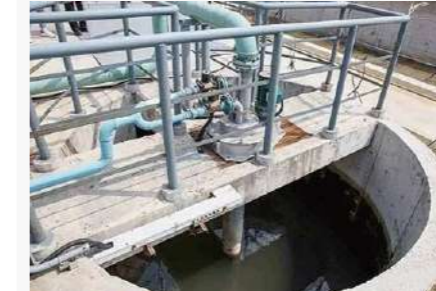
Centrifugal Sand Settling Tank
