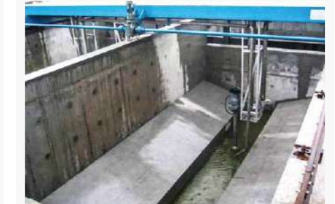
Flow-type Sedimentation Tank
